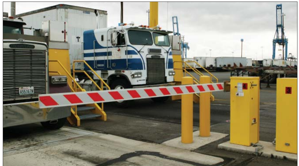
StrongArm 20 with 18' aluminum barrier arm installed at one of North America's leading seaports: Port of Tacoma
