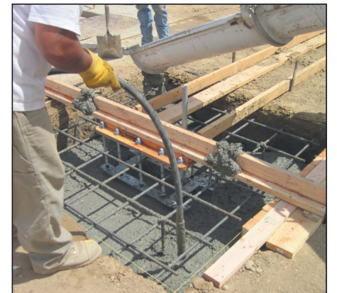
This photo shows concrete reinforcement being poured into the StrongArm M30 foundation. The crash test capped 18 months of design and development for HySecurity's first crash product.
