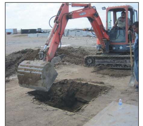
A backhoe is used to excavate where the extremely heavy duty base of the StrongArm M30 will be installed.
